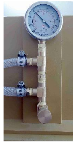
Figure 3 Manifold and bleeder valve
