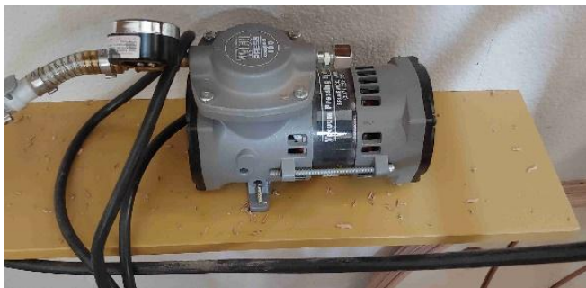
Figure 4 Vacuum pump on the wall.
